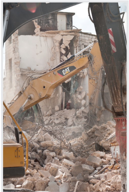
House demolition in Sheikh Jarrah neighbourhood in East Jerusalem, January 2011. (Photo by Ridvan Yumlu)
